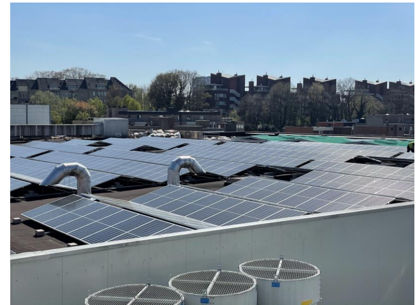
Shopping 1 Genk: 1.765 solar panels installed, 450 kWp capacity. This is about 20% of the shared services electricity consumption
